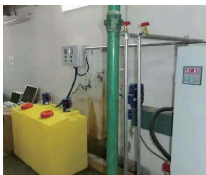
泳池药剂添加及空调制冷 Pool Sterilization
